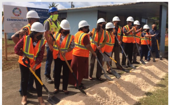
GHC held a groundbreaking ceremony for Phase I of the Lada Gardens Renovation Project led by Governor Lou Leon Guerrero and Lt. Governor Joshua Tenorio.
